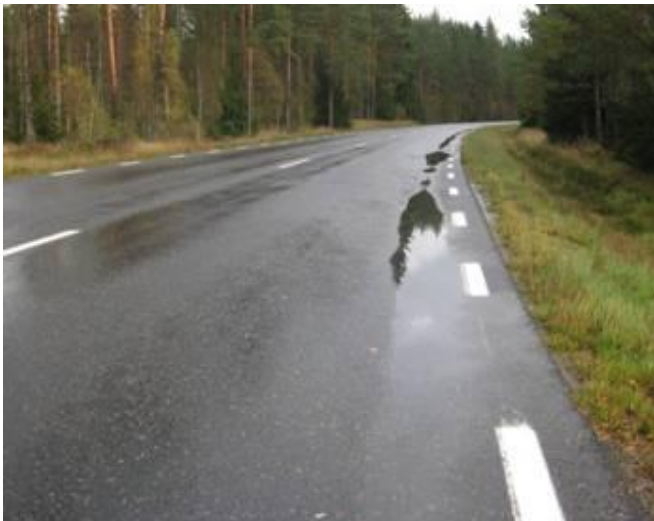
Rutting (plastic deform.)
