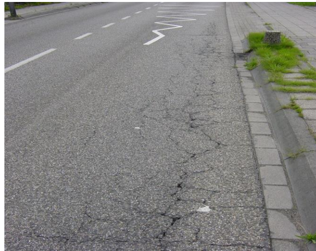
Fatigue cracking (bottom-up)
