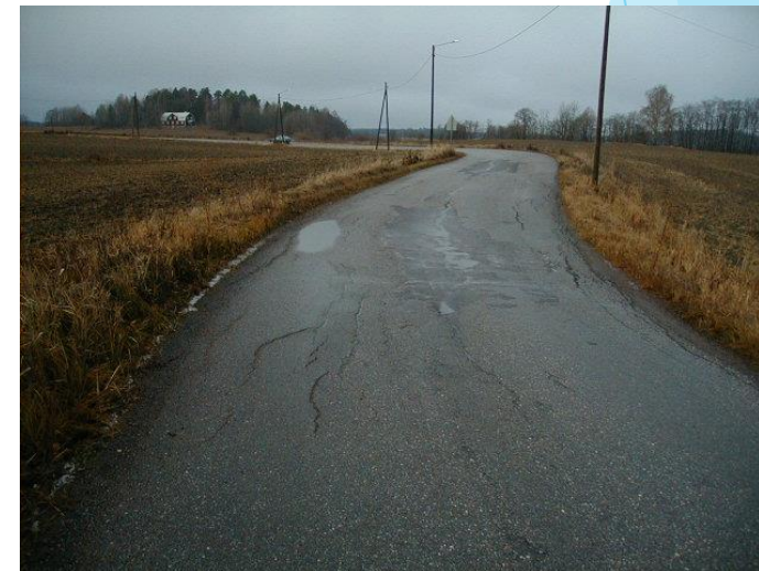
Frost actions & frost heave damage
